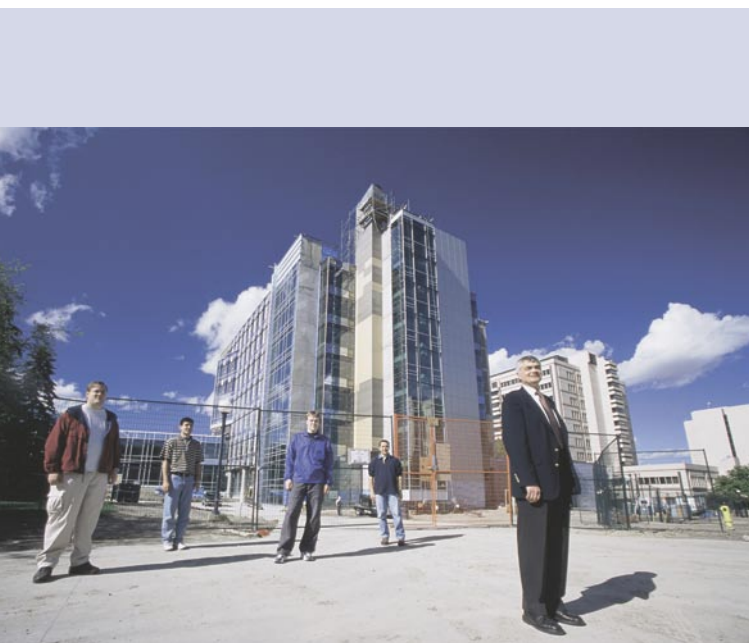
Graham Jullien and research team members during construction of the new Calgary Centre For Innovative Technology building on the University of Calgary campus
